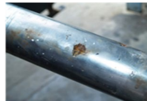
Deep pitting on bearing surface
