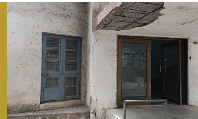
Dilapidated condition of several external elements
